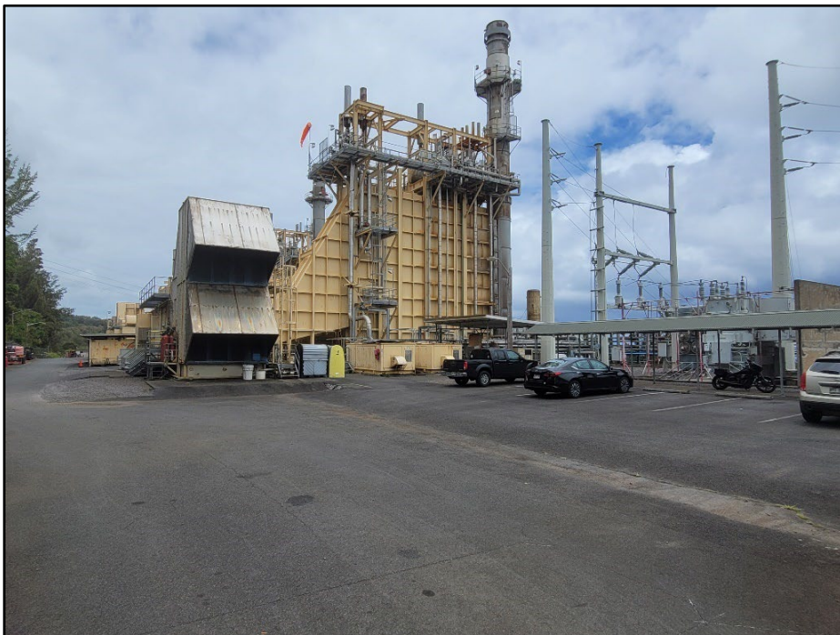
Figure 14. Photo overlooking plant facilities; view to northwest
