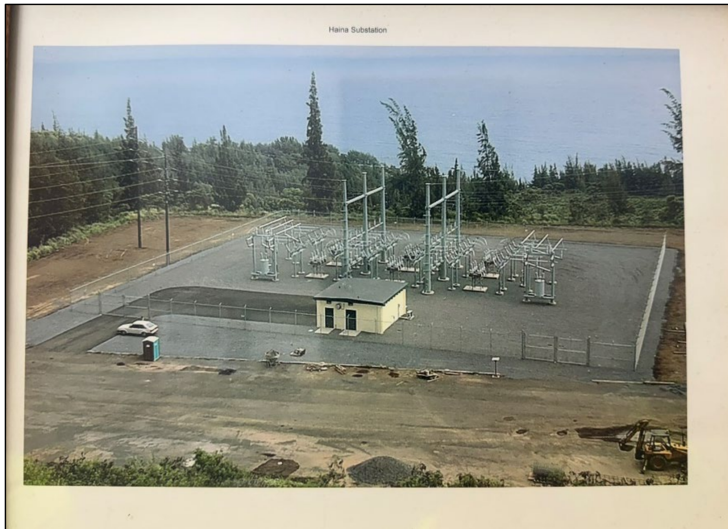
Figure 26. Photo on display at the existing Hamakua Energy Plant, showing the Haina substation shortly after completion ca. 2000; view to north
