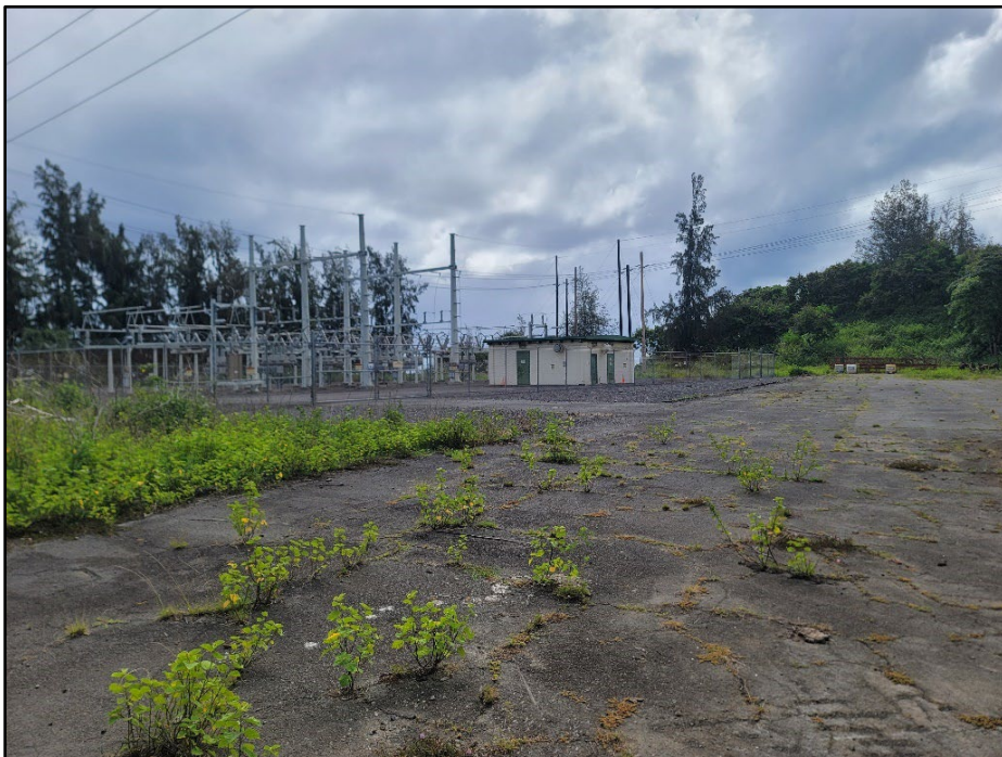
Figure 20. Photo overlooking the existing Haina Substation and adjacent asphalt lot (proposed battery storage site); view to northeast
